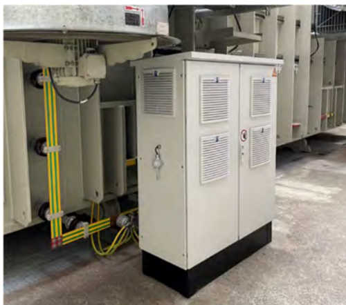
Figure 3: The DC Mitigator installed in the connection from Neutral bushing to substation ground.
