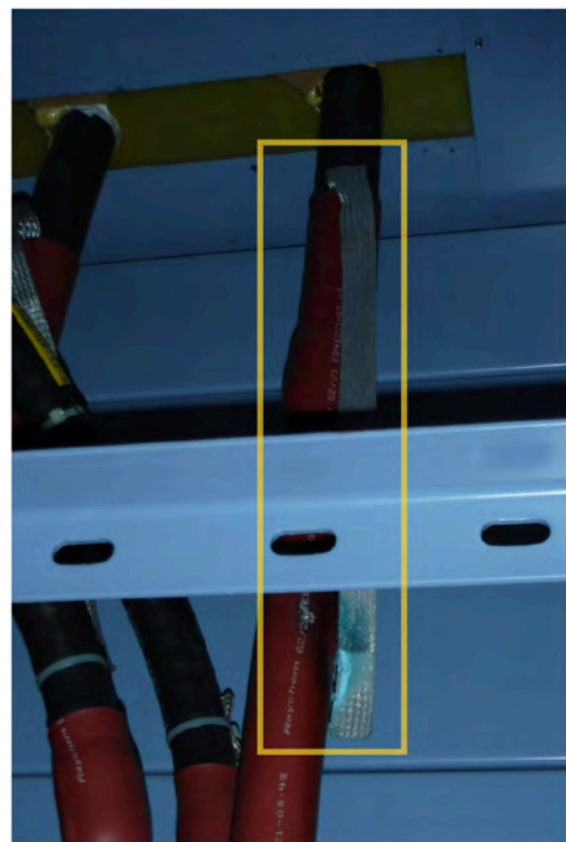
Figure 11: Grounded copper tape
